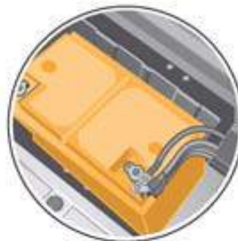
Fuse holder (SA), on right-hand side of battery, visible only following removal
