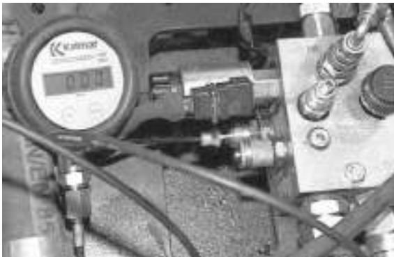
Measuring outlet, accumulator pressure
