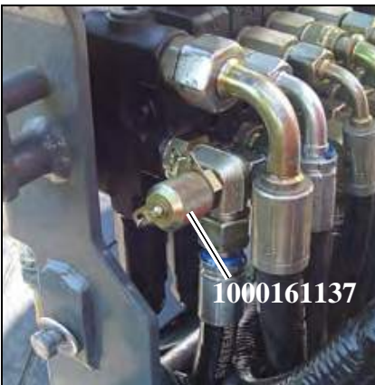
Fig. 29: Secondary pressure limiting valve measurement connection
