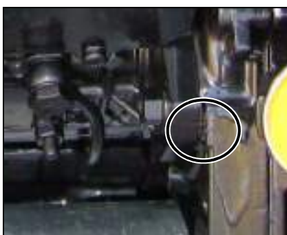
Fig. 35: Mark on pump housing
