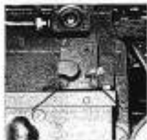
Fig. 26 - Cracking distributor upper cover screws
