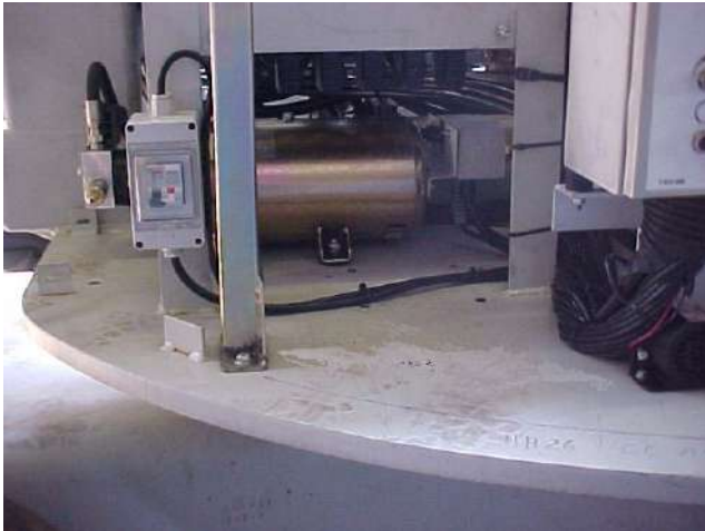
Photo 11 - Built-in generator and
