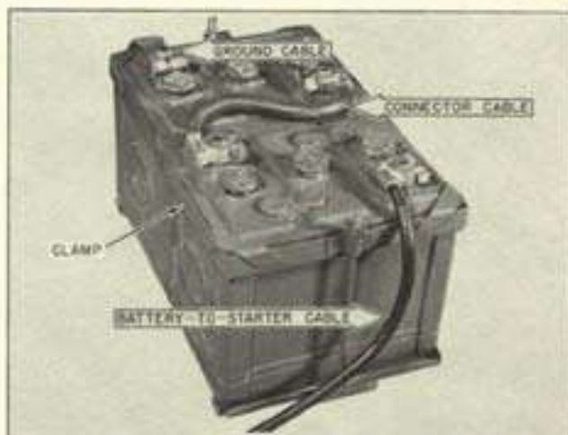
Figure 4-5 Batteries Connected For Diesel Installation
