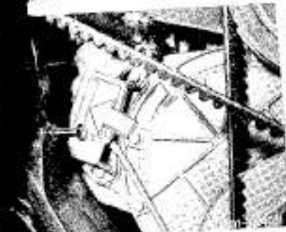
Operating hour counter at front of engine
